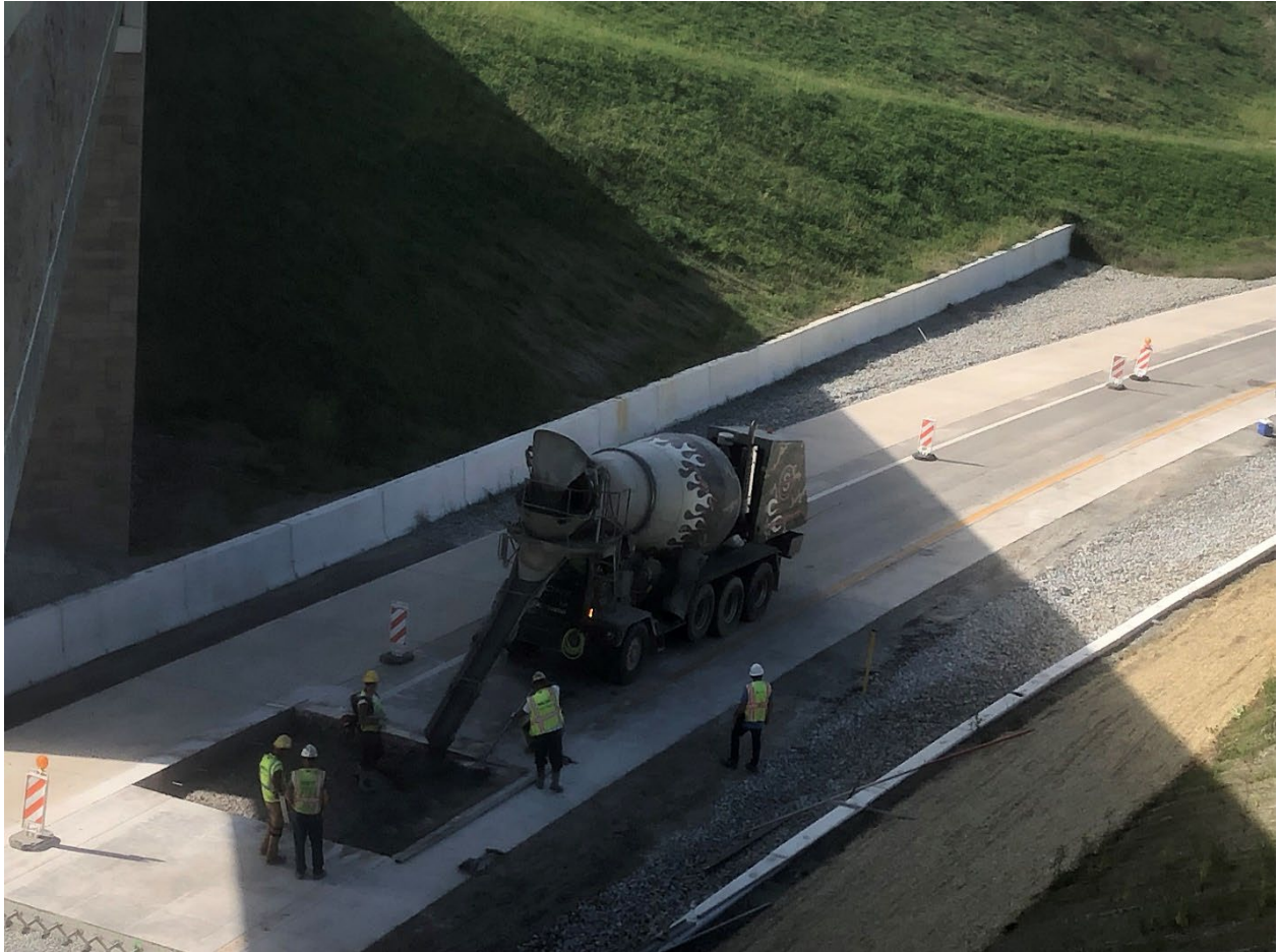
Section: 55C2-1 — Pictured: Concrete pavement slab replacement on Ramp 79N to 576W
