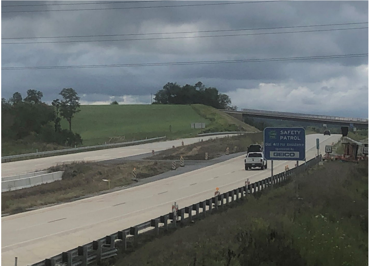
Section: 55C2-1 — Pictured: Emergency crossover on PA Turnpike 576
