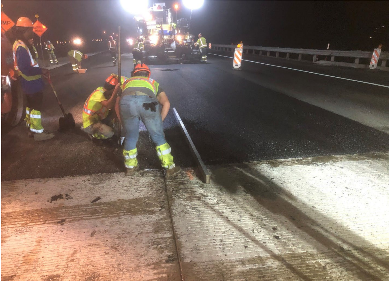
Section: 55C2-1 — Pictured: Straight edge testing asphalt at bridge approach on I-79 southbound
