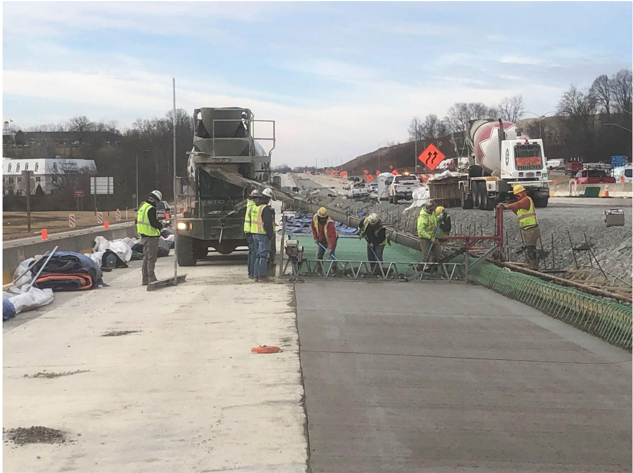
Section: 55C2-1 — Pictured: Placing concrete for the moment slab on I-79 NB.
