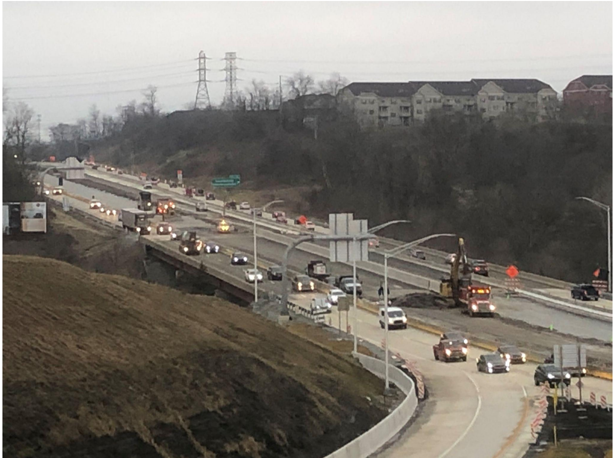
Section: 55C2-1 — Pictured: Excavation to remove existing roadway and backfilling of undercuts with No. 1 stone, I-79 median
