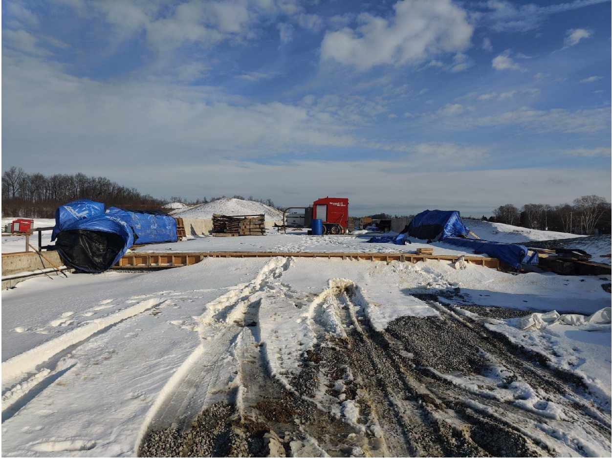
Section: 55C2-1 — Pictured: Cold weather curing SB-294 moment slab parapets, insulated blankets and ground thaw heaters
