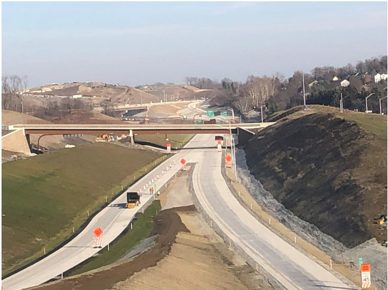
Section: 55C2-1 — Pictured: Opening of the ramp from Morganza Road to PA Turnpike 576 westbound
