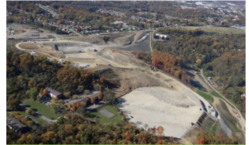
Aerial view of excavation for New Highway at Camp Hollow and Curry Hollow Roads.
