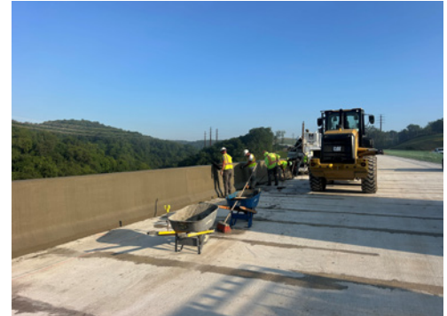
Slipped formed bridge parapet - bridge over New England Road.
