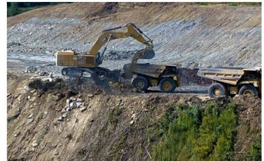
A large excavator loads road trucks at the new PA Turnpike 43 south to the Jefferson Boulevard exit ramp.
