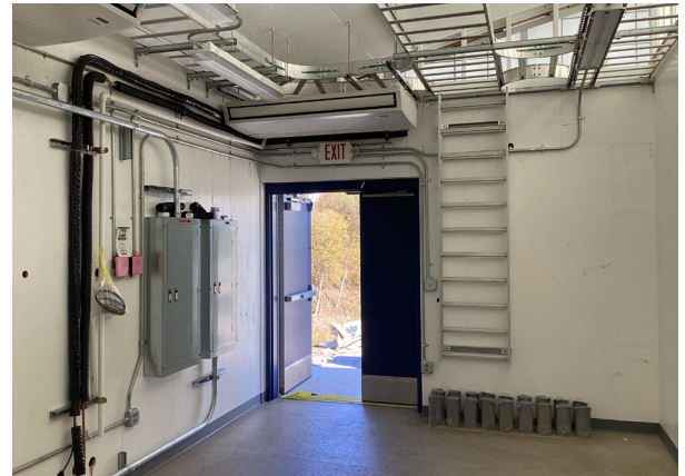
Toll facility building ready for data servers.
