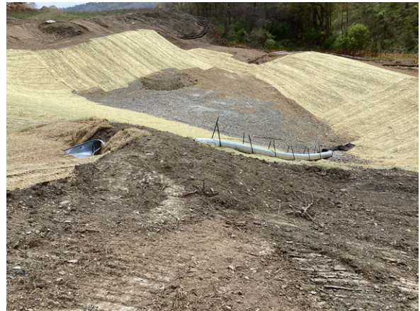
Work continues on a sediment basin for the 53A1 Section of the Mon/Fayette Expressway.
