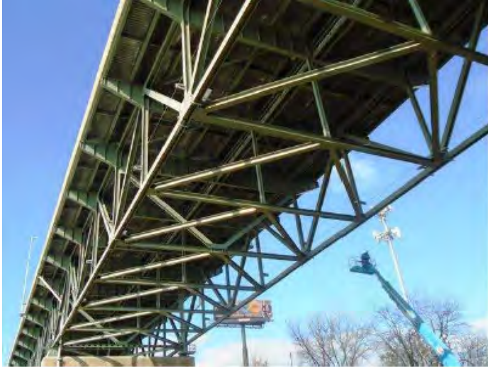
Photo 5: Steel Continuous Deck Truss spans (Span 14 shown), looking northeast (Photo: ATANE Consulting, 2022)
