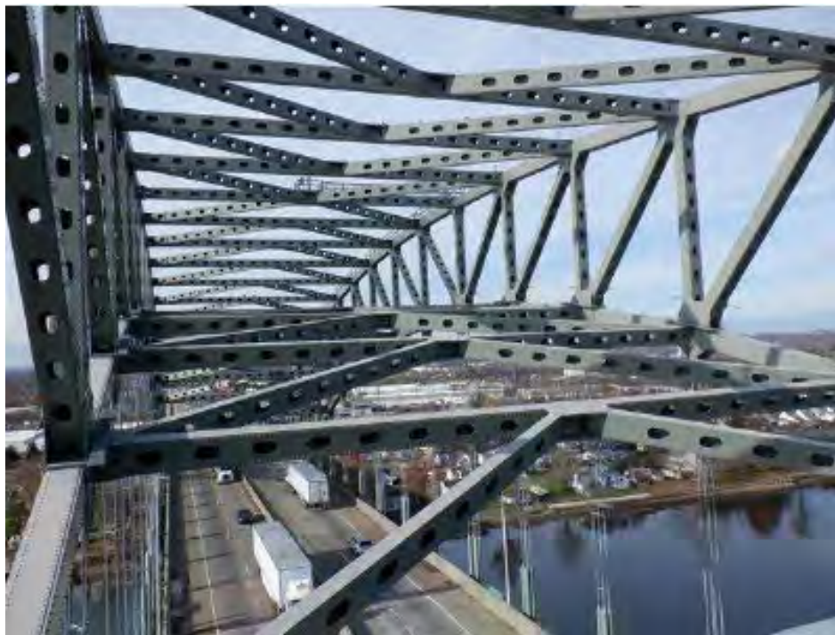
Photo 4: Three-span Steel Continuous Warren Through Truss spans (Spans 18 to 20 shown), looking east (Photo: ATANE Consulting, 2022)
